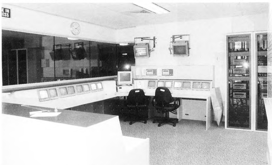
The operation of the watch-house is managed from the control console which directly overlooks the pre-charge holding and person-at-risk cells.
