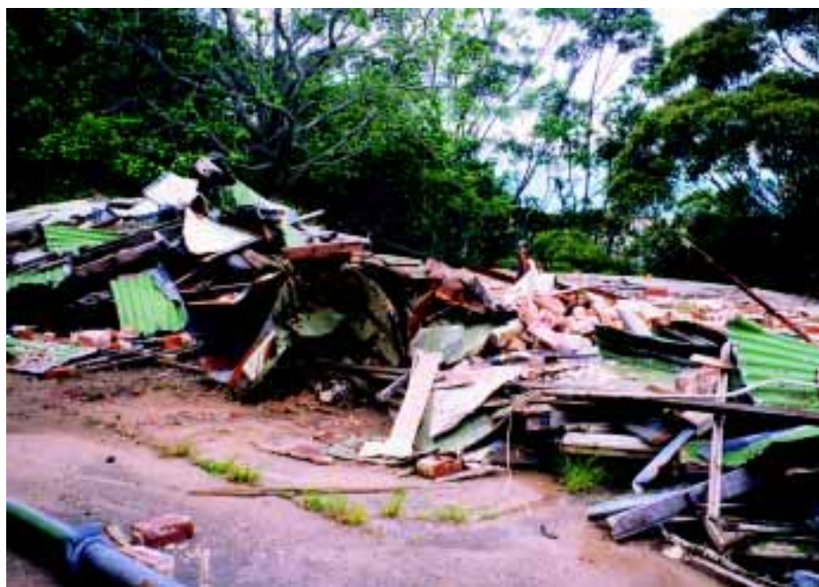
This old mine building on Mt Keira was destroyed by a debris flow during the Wollongong floods in August 1998.
