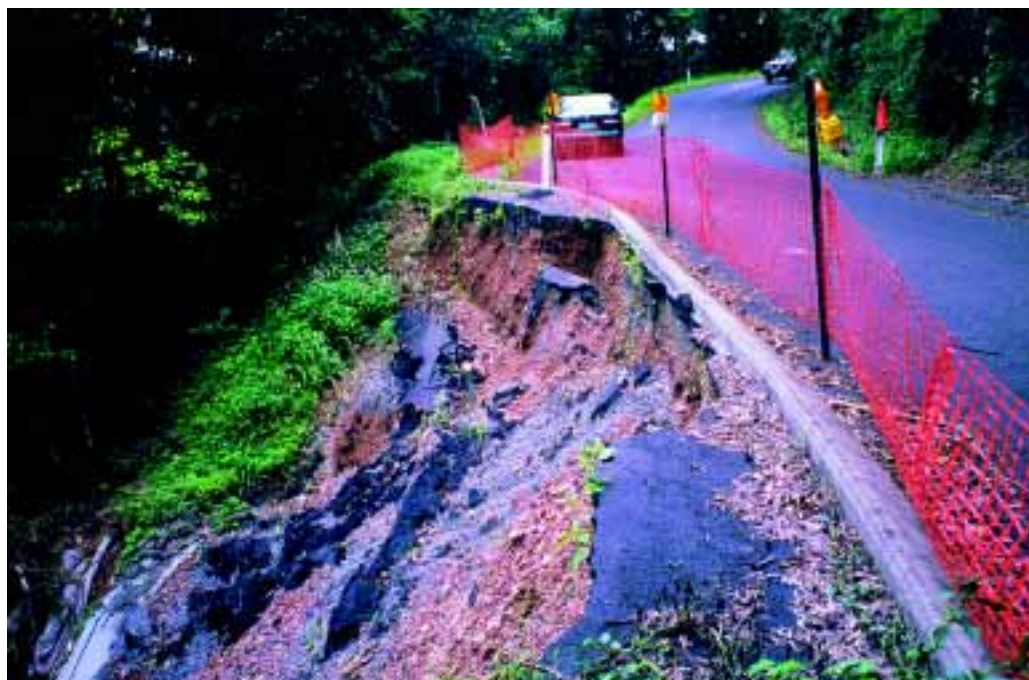
This landslide, on Lake Morris Road near Cairns, was triggered by heavy rain in March 1999.
