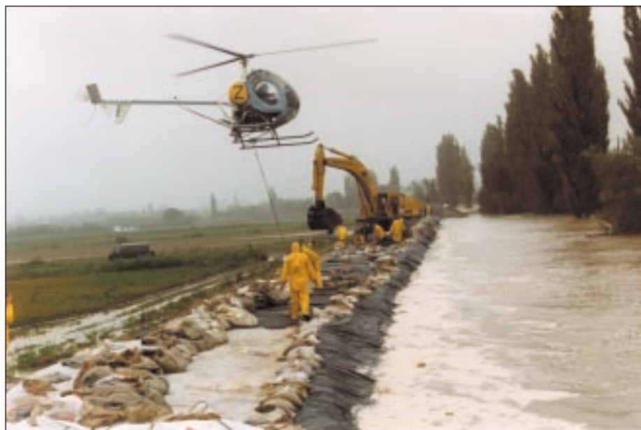
Figure 4: The Hawke's Bay Regional Council repairs the Ngaruroro stopbank with dandbags during Cyclone Bola in 1988. This photo also shows how stopbank schemes protect horticultural land in Hawke's Bay.
