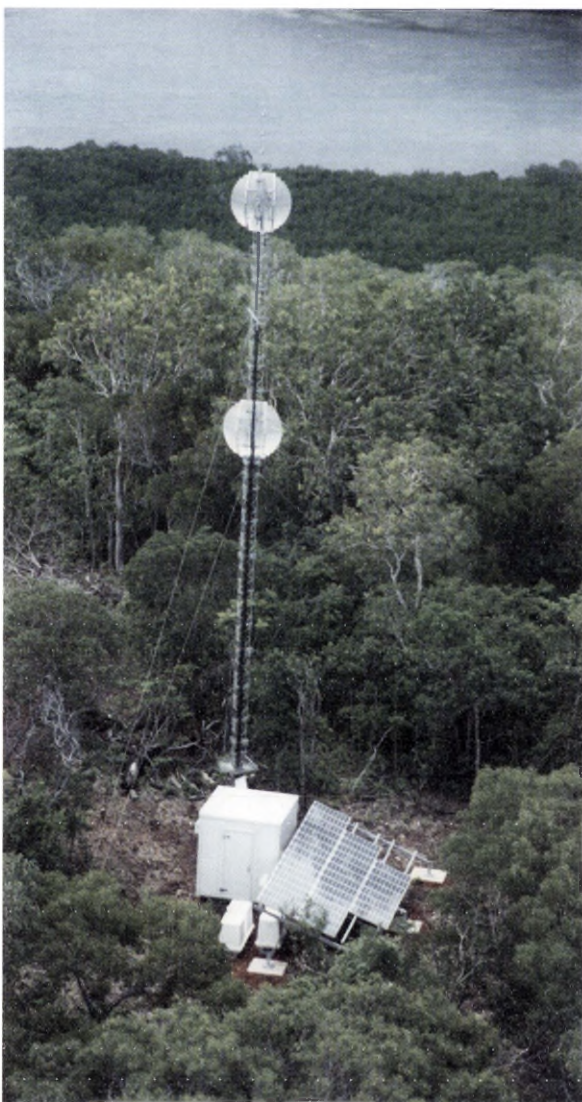
A radio mast located at Banks Peak on Moa Island in the Torres Strait has assisted in bringing secure communication to the region.
