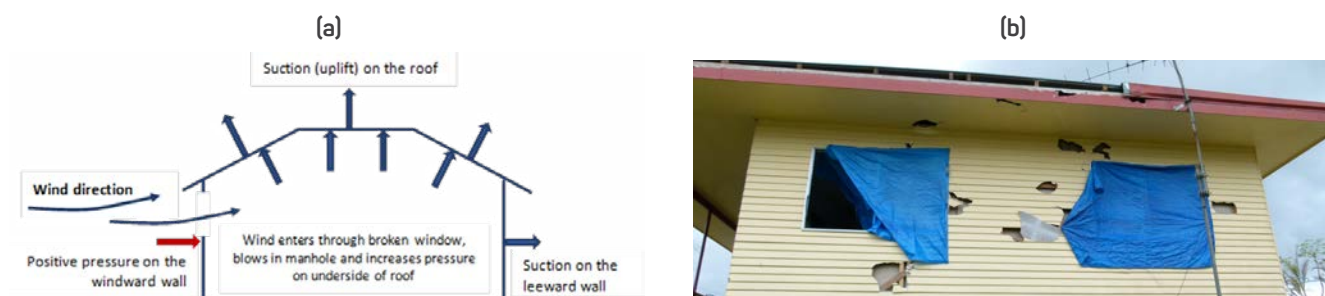
Figure 2: (a) Wind pressures on building and (b) example of damage caused by debris during a Tropical Cyclone Seroja.
